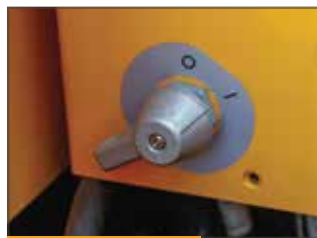
BATTERY DISCONNECT SWITCH
